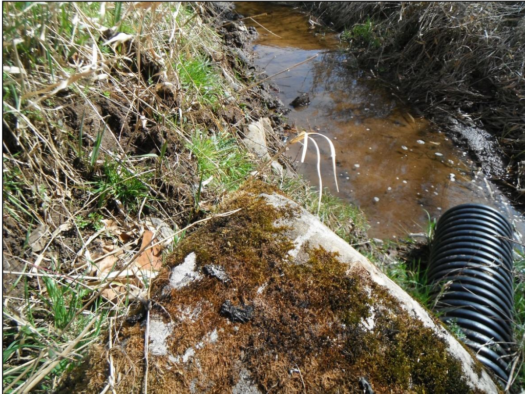
Figure 19: Spraint above new drainage outfall pipe
