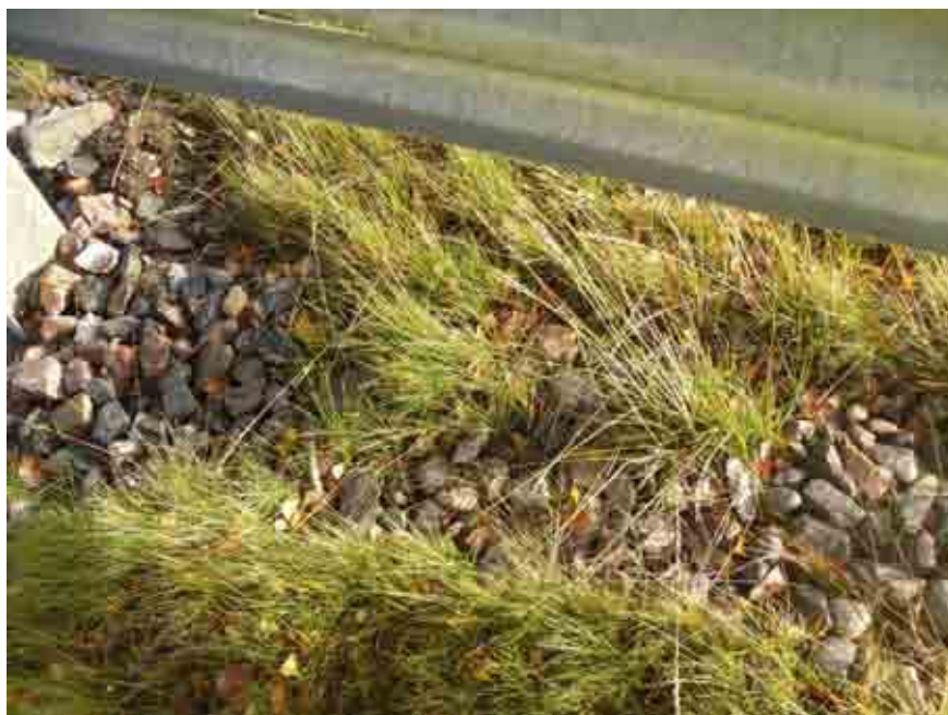
Figure 2 Weed growth in filter drain along Northbound Carriageway
