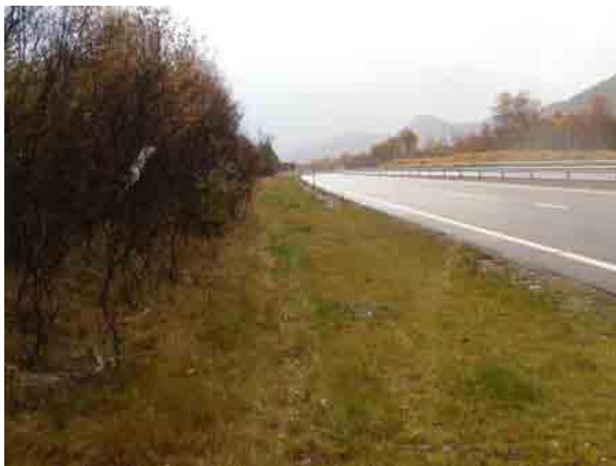
Figure 4 Gap in filter drain along Southbound Carriageway
