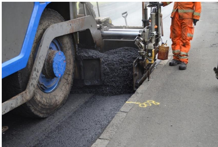
Figure C-2 Close up of asphalt surfacing (TS2010)
