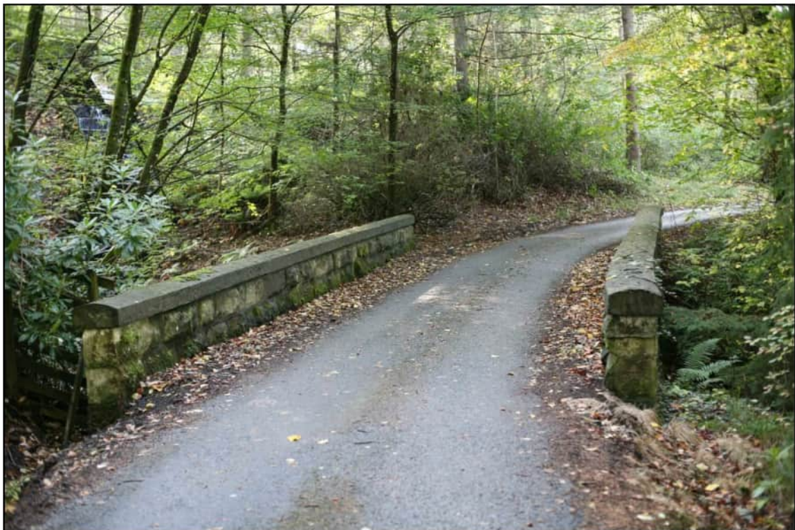
Photograph 14.2: Birnam Burn Bridge (Asset 3), a Category C Listed Building, showing the stone parapets and western drive, facing west
