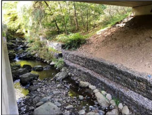
Photograph 10.3: Incheon Burn (WF8) – upstream view of restored section underneath A9 bridge (example of a medium water feature).
