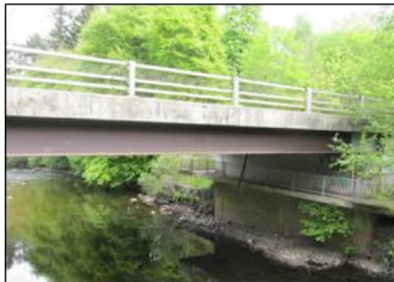
Photograph 7.2: River Braan Crossing – taken from the foot bridge over the River Braan adjacent to the northbound carriageway of the existing A9
