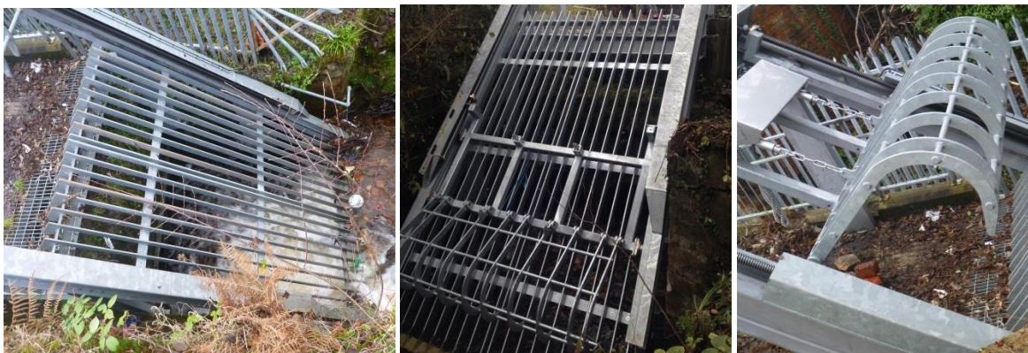
Figure 3. Automated self-cleaning trash screen at Crescent Street culvert inlet.
