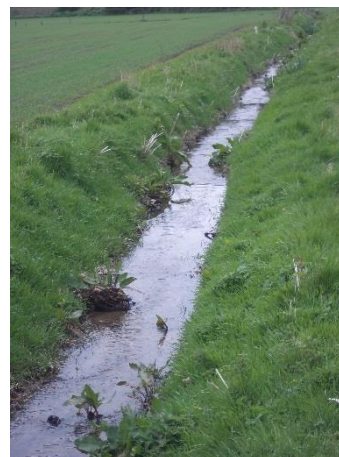
Photograph 7b: Straight planform and embankment downstream of the existing A9 (looking downstream)
