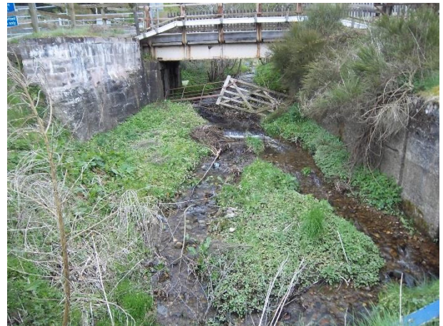
Photograph 8b: Section of bank reinforcement immediately downstream of the highland railway (looking upstream)
