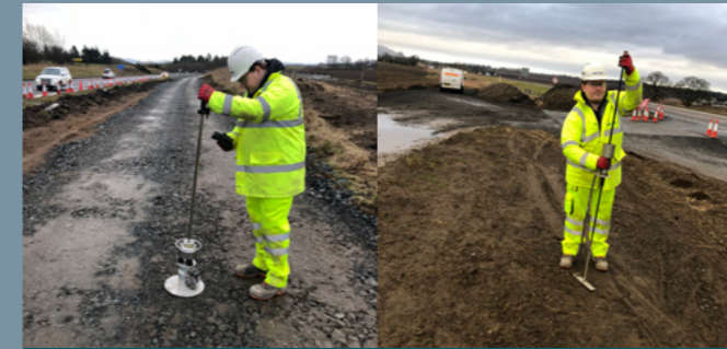
James is completing a Light Weight Deflectometer (LWD) test to determine ground stiffness/check compaction
