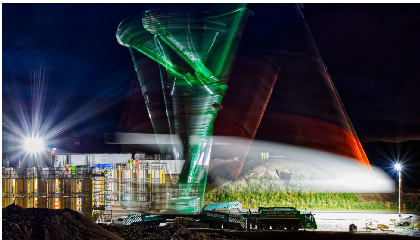
A long exposure captures the 750-tonne crane lifting the 15 concrete beams over the existing carriageway
