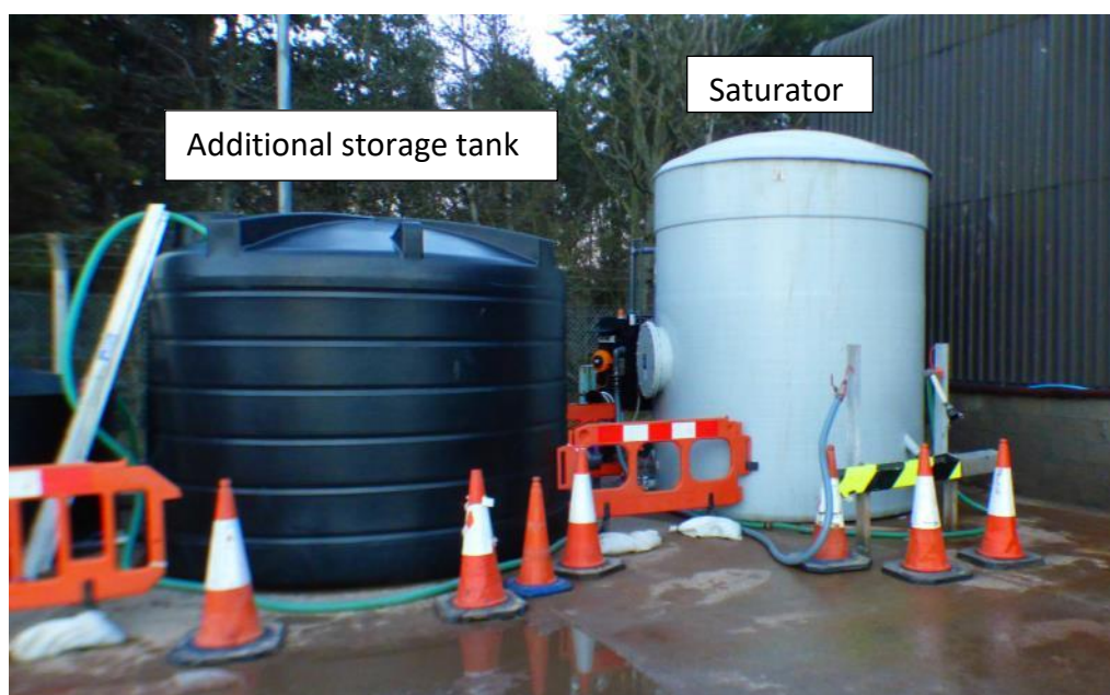
Figure 4. Saturator and brine storage tank
