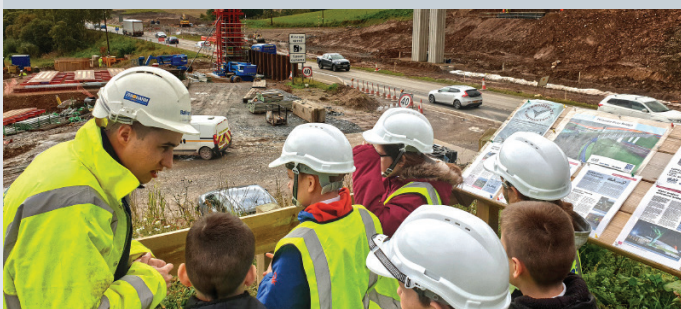
Structures Sub Agent, Gary Cameron, talking to primary seven pupils about the construction of Pitlandie Overbridge
