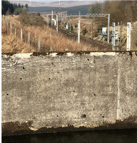
Figure 38. The surrounding walls of the aqueduct are in poor condition.
