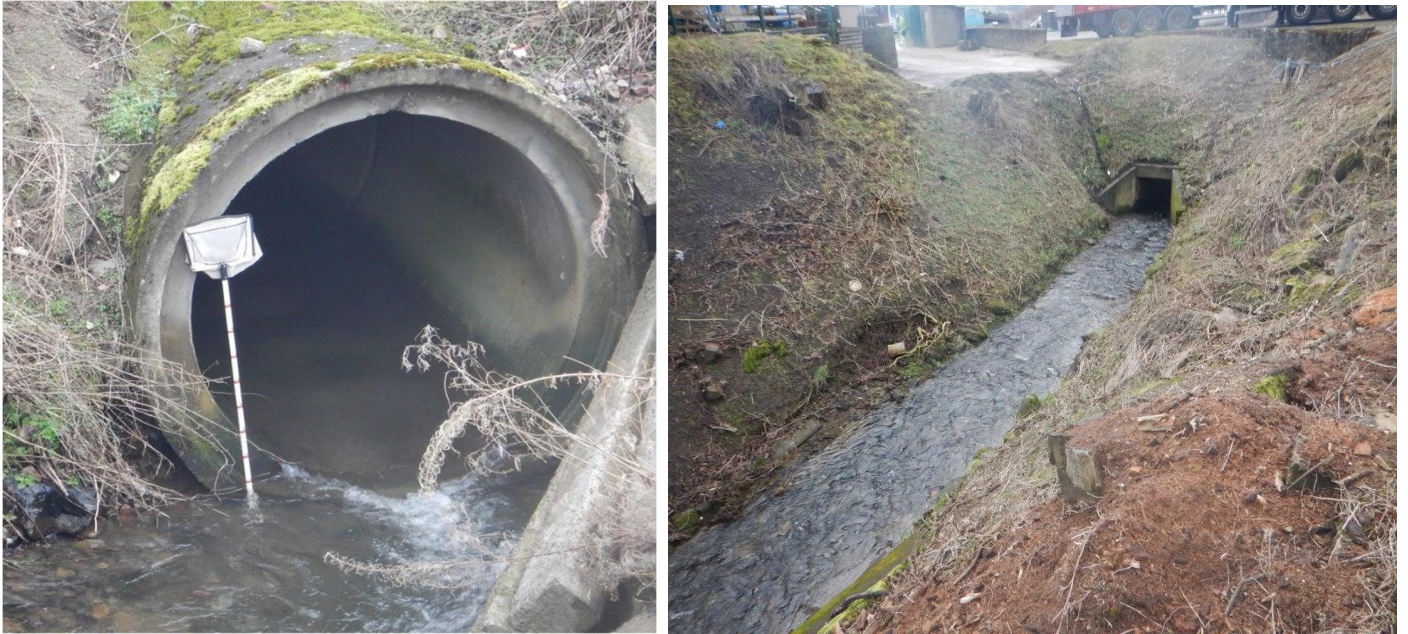
Figure 30. The downstream outlet on the left and the upstream inlet on the right (Culvert 2).
