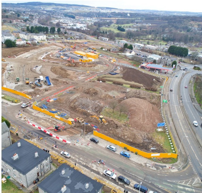
Progress showing utilities crossing Manor Avenue near to the junction with North Anderson Drive
