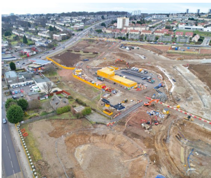
Foreground showing the progress on the Sustainable Urban Drainage System detention basin with the utility trench works on the right-hand side, also shows the new road alignment taking shape behind the Farrans site accommodation
