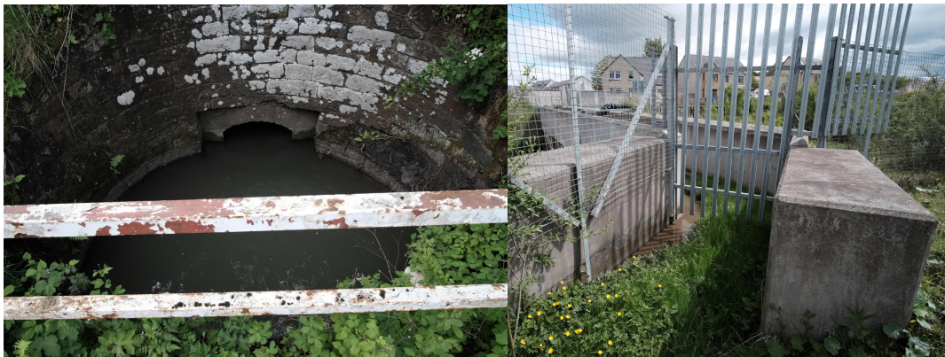
Figure 2-4 (A) Outfall from the Union canal culvert and (B) Inlet to the railway aqueduct.
