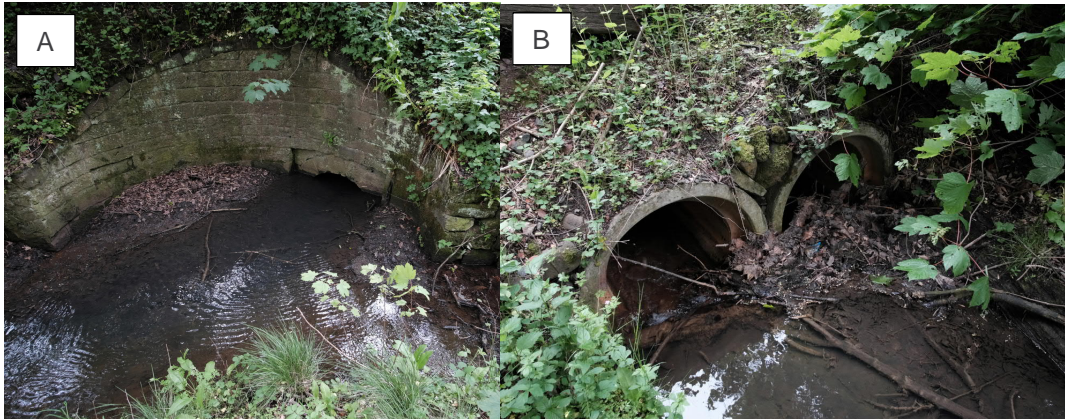
Figure 2-3 (a) Downstream of the Union Canal Culvert and (b) upstream of the two culverts along the Swine Burn
