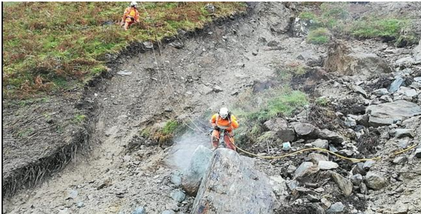
Significant channel debris
