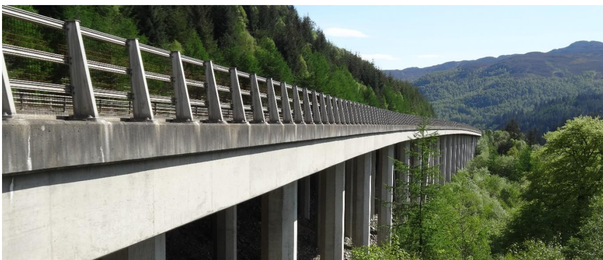
Figure 50 – the elegant structure at Killiecrankie has a high potential for bat roosts.
