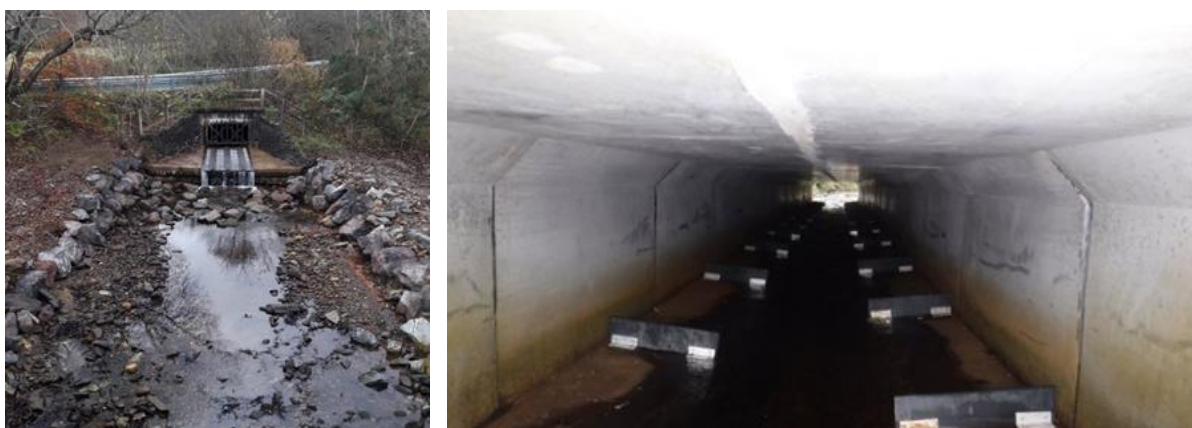
Figure 48 & 49 – the driver for works at this location was for scour protection but opportunity was taken to improve the culvert for fish (and eel) passage by installing fish tiles on the new culvert apron and baffles within the structure.
