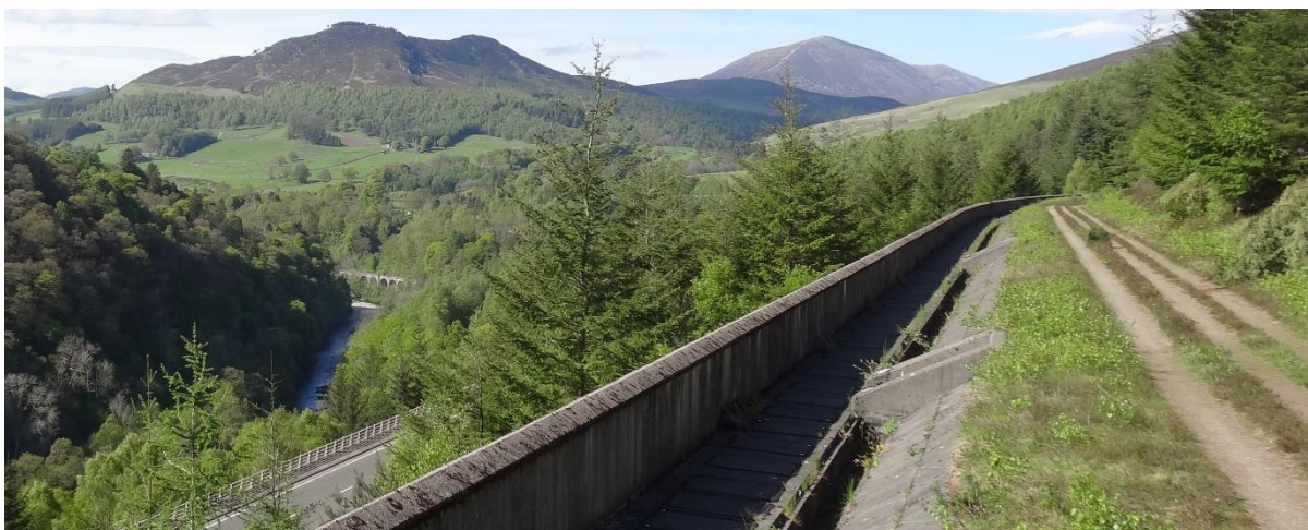
Figure 51 – Above the viaduct on the A9 lies a significant retaining wall that supports the rocky slopes of the Pass of Killiecrankie.
