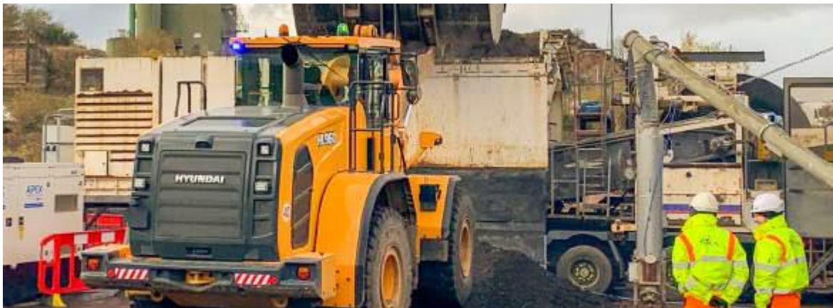
The worn-out road material was transported to a nearby mobile plant where it was reprocessed for reuse in the project.
