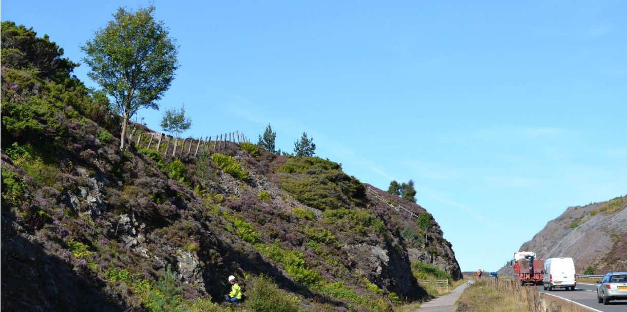
Lot 3 - 'Site surveys alongside National Cycle Network Route 7 and the A9 at Slochd Summit'
