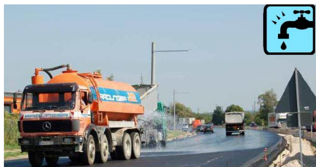
Figure NG 2.4: Watering of surface to avoid sticking of bond coat to tyres
