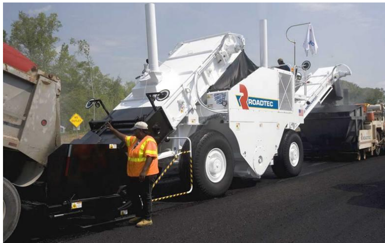
Figure NG 2.2: Example of shuttle buggy in operation
