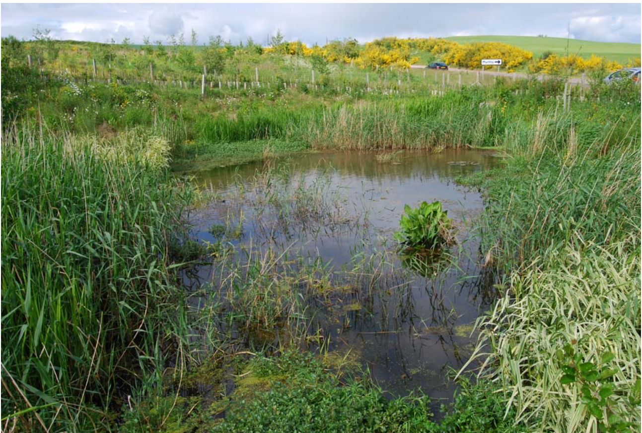
Existing road drainage treatment pond (SUDS), alongside the A9 at Bankfoot Junction
