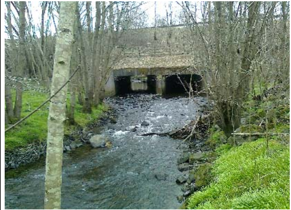
Photograph 2: Culvert No.1 – Looking upstream towards the outlet of the existing Shochie Burn twin cell box culvert under the A9 single carriageway embankment.
