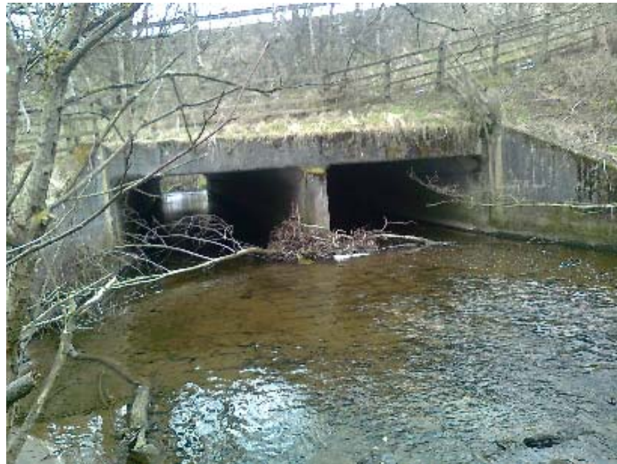
Photograph 1: Culvert No. 1 – Looking downstream towards the inlet of the existing Shochie Burn twin cell box culvert under the A9 single carriageway embankment (upstream side to be extended).
