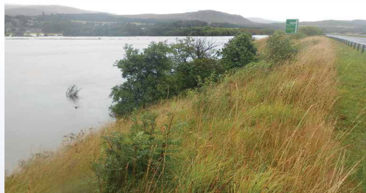
View of flooding at River Spey, looking north towards Kingussie, August 2014
