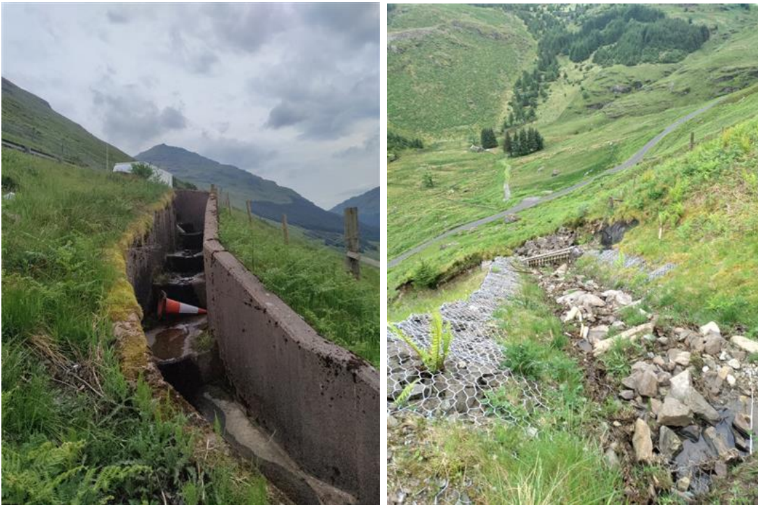
Plate A19.3.8 Examples of downstream built cascade and bank protection to watercourse A83_ML_029_000 (left) and A83_ML_023_000 (right) (Dated: 22 May 2024)
