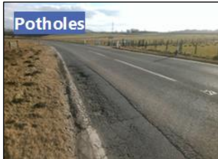
Figure 2.12: Images of defects shown to respondents
