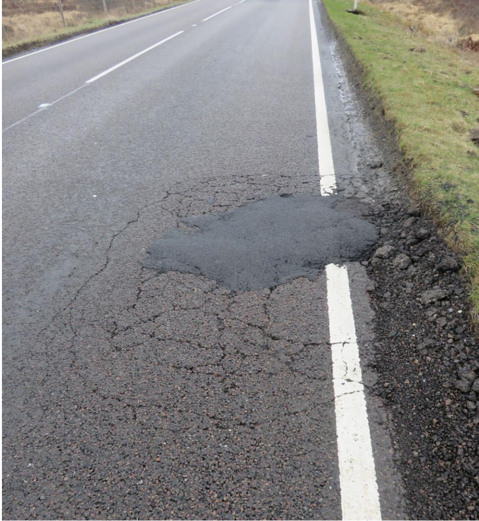
Figure 4-2 - Structural failure noted on A82 at 2.5 years old
