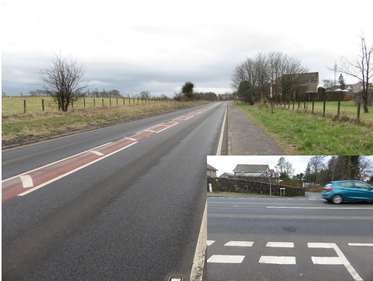
Figure 3-3 - A737 Beith with single pothole (18 months old)
