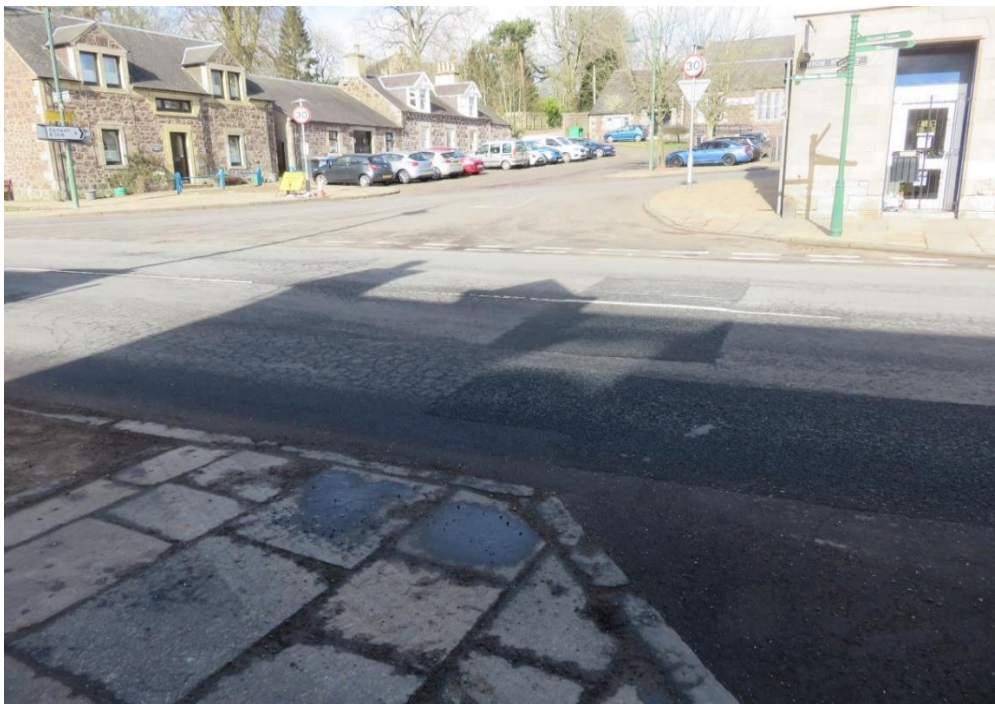
Figure 4-4 - Alligator cracking and remedial treatment at A702
