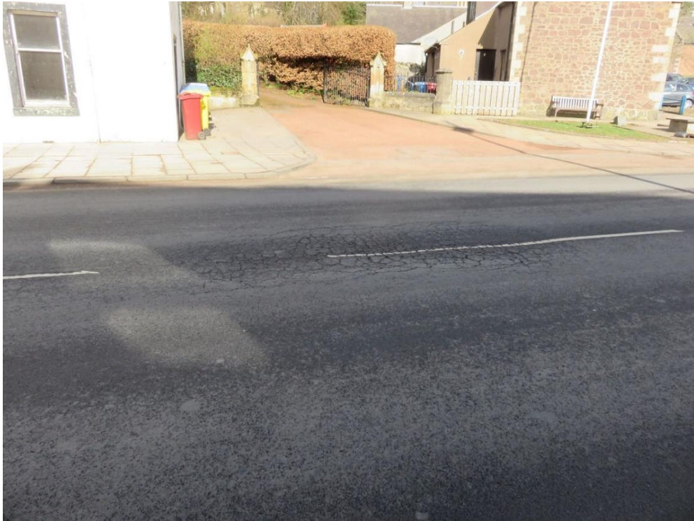
Figure 4-3 - Structural failure on A702 after 22 months
