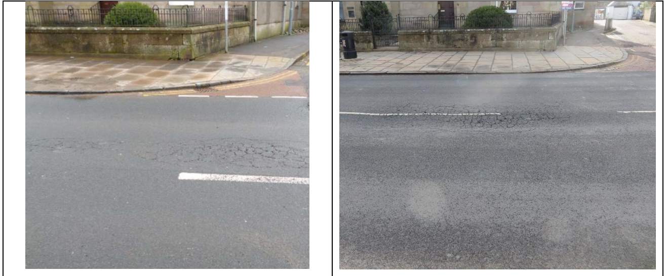
Figure 3-10 - Structural rutting before treatment (left, 2018) and after treatment (right, 2021)
