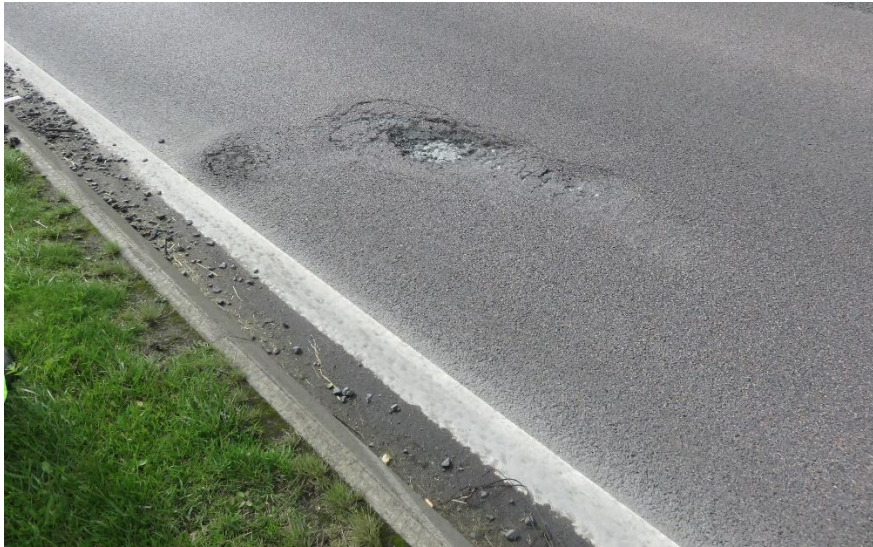
Figure 1-1 - Early life defect on one-year-old surfacing
