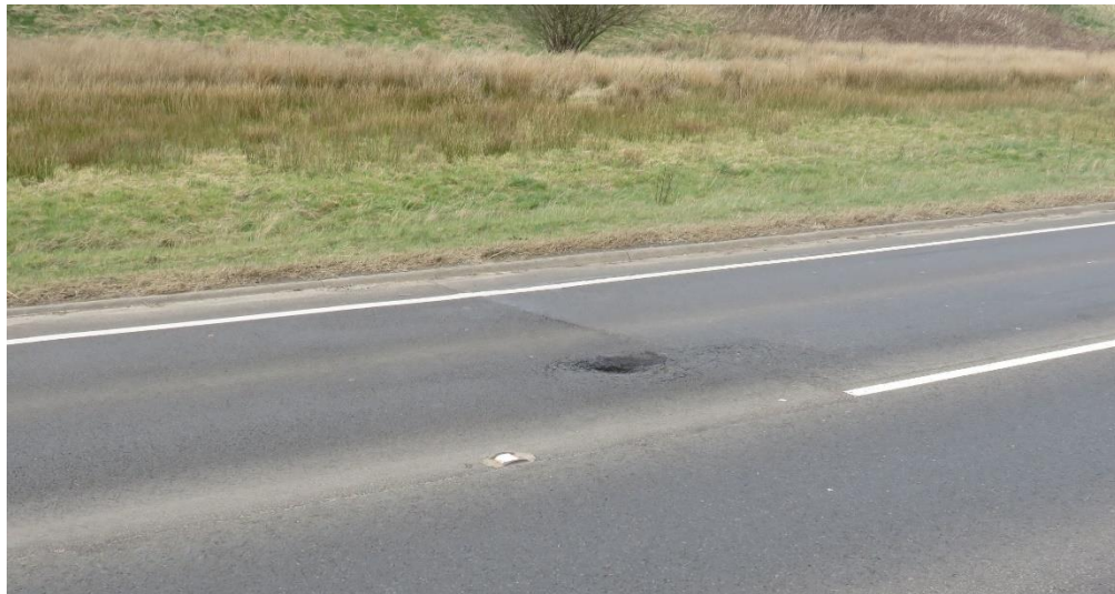
Figure 3-6 – Defect on A77 near Drumellan Farm (2021)
